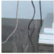
Several inches of water in a basement with a broken sump pump. (photo, Terry Brennan)
