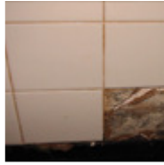
Mold growth under ceramic tiles in a bathroom. (photo, John Martyny, Ph.D.)
