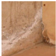
Water in the ground has seeped through the concrete walls of the basement, leaving white mineral deposits on the walls. The water has evaporated into this basement, increasing humidity. Mold is growing in some areas. (photo, John Martyny, Ph.D.)
