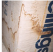
Water stains in basement. (photo, Terry Brennan)
