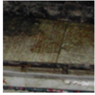
Mold (and dirt) beneath refrigerator due to chronic drip-pan overflows. (photo, Terry Brennan)
