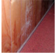
Mold on wooden paneling. (photo, Terry Brennan)
