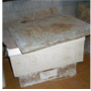
Mold growth on fiberboard shelf (left) and on cardboard boxes (right) due to high humidity. Water is condensing from the basement air, which is at approximately 90% relative humidity (RH). (photo, Terry Brennan)
