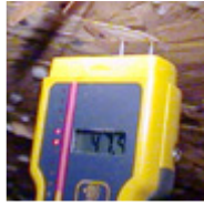
Moisture meter and moldy roof sheathing. (photo, Terry Brennan)
