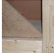
Mold on basement ceiling resulting from chronic high humidity (>90% relative humidity[RH]). (photo, Terry Brennan)
