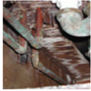
Moisture damage and mold growth under bathtubs. (photo, Terry Brennan)
