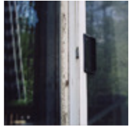
Mold on air seal on sliding glass door.
